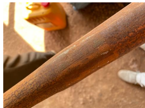
(f) Squashed pipe from lifting (most likely not correct grade) Source: Richard Carter.
