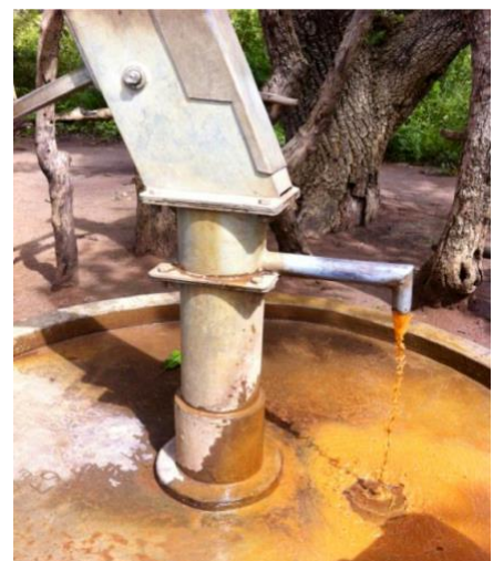
FIGURE 4 RED, IRON-RICH WATER BEING PUMPED
