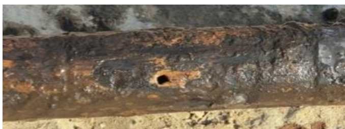
(a) Riser pipe corrosion in Zambia Source: SOMAP3, 2013.
