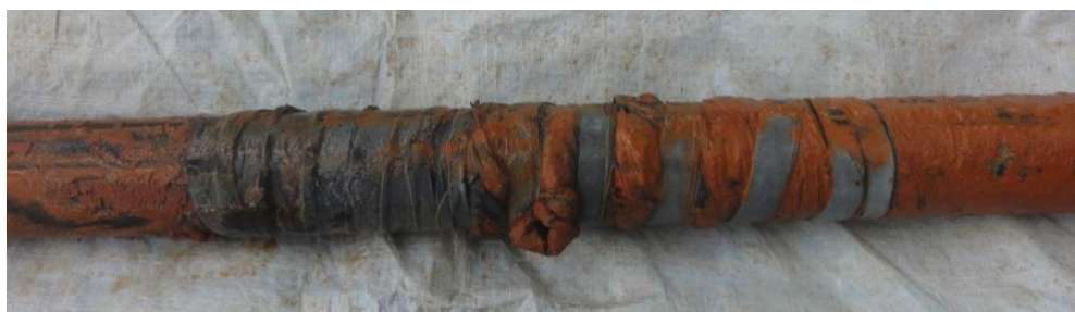
FIGURE 8 CORRODED RISER PIPE WITH BIOFILM AND REPAIRS USING AN INNER TUBE IN AMURIA, UGANDA Source: Richard Carter.
