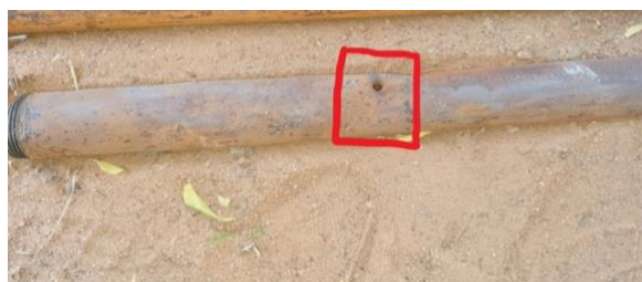
(b) Riser pipe corrosion in Nigeria Source: Olajide Oyetunde.
