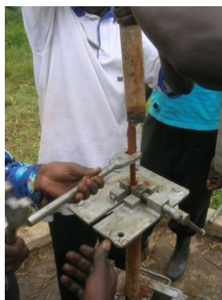
(b) Removal of corroded pump rods and riser pipes in Hoima District, Uganda, 2012 Source: Larry Bentley.
