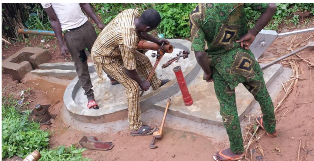
FIGURE 9 CHANGING RUSTED CYLINDER IN OSUN STATE, NIGERIA Source: Olajide Oyetunde.
