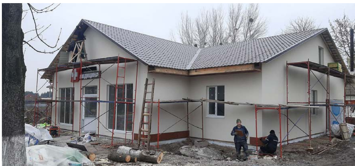
© DESPRO NGO – Reparation works of the Primary Healthcare Center in Hurivshchyna village.
